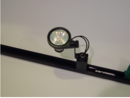
Conforming – low voltage “green”
