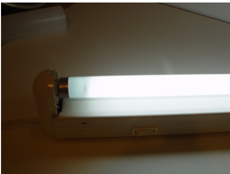
Non-conforming – exposed bulb
